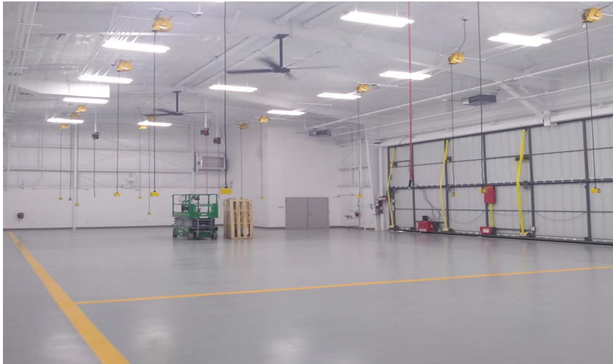
Aviation Lab w/Compressed Air Stations
